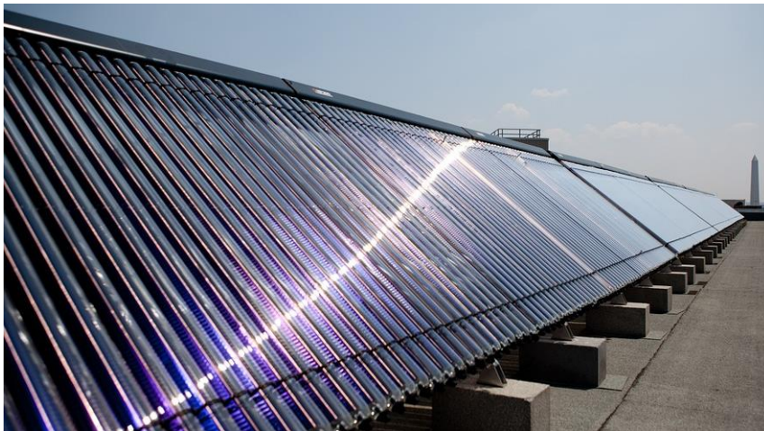
Figure 3: Solar Water Heating Panels example.
